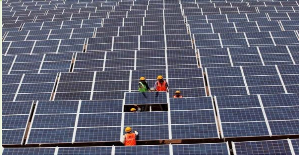
600MW Solar Farm at Patan, Gujarat
